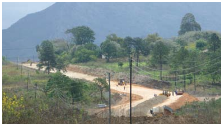
Changing landscape ... new road construction to connect the Matsapha airport with the southern Matsapha Industrial Estate.
